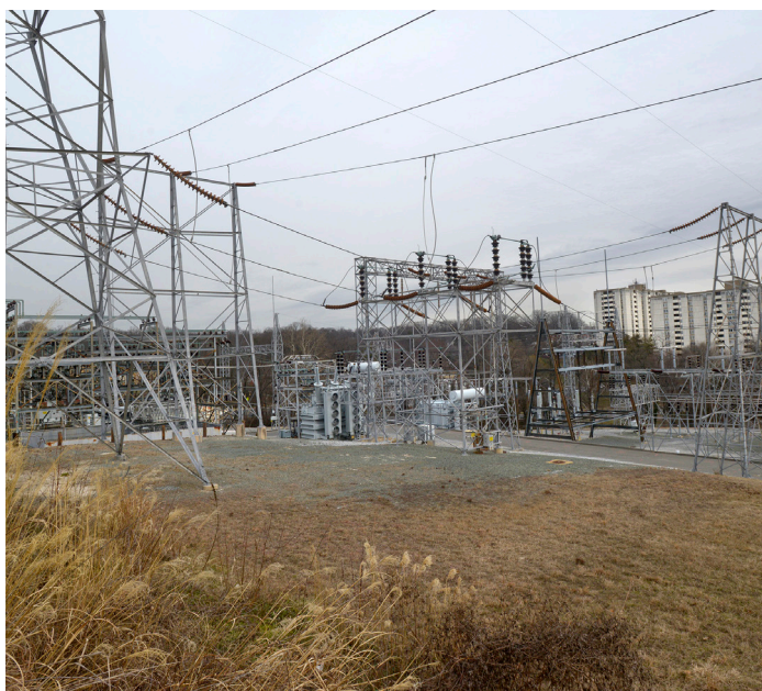
Current Takoma Substation
